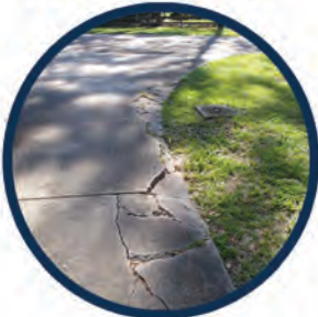
EROSION & DRIVEWAY HEAVING
