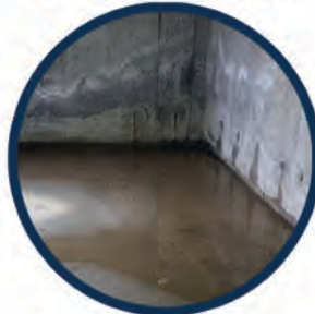
LOWER LEVEL FLOODING
