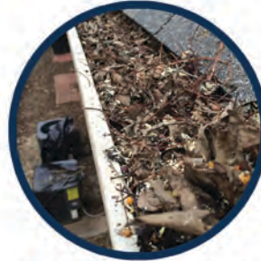
BLOCK DEBRIS BUILDUP
