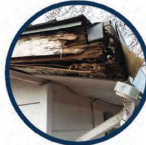
FASCIA ROT & WATER DAMAGE
